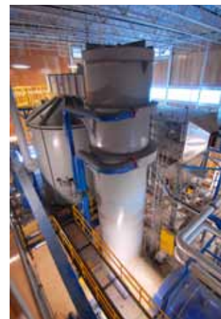
The UNBC plant gasifies sawmill residue to heat water that provides heat for the Prince George campus. Photo courtesy of UNBC.
